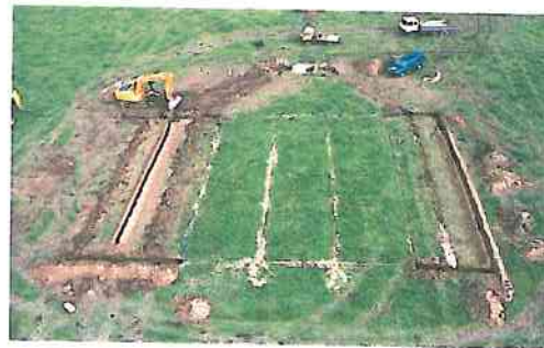
Drainage plots constructed to measure nitrate leaching from heavy clay soils on the South Block of LUDF.
